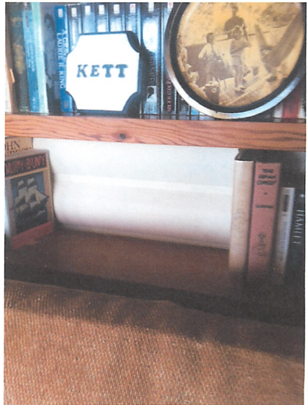
Portion of old exterior wall of cabin, now behind bookcase in sleeping porch addition and painted
