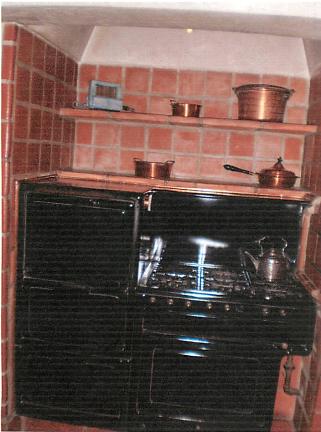
Nine Burner, Four Oven Stove in Kitchen
