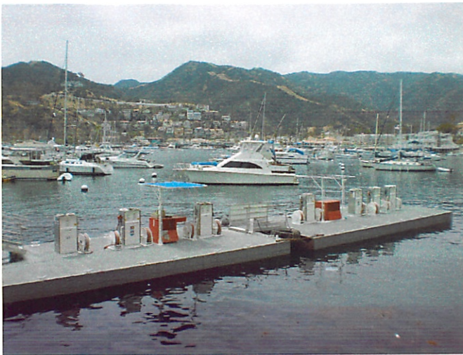
A Floating Gas Station on the Bay
