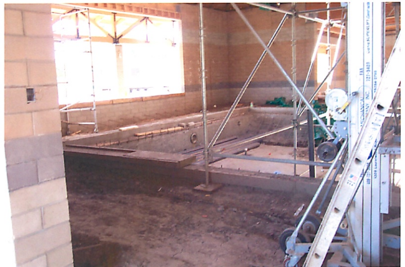
060511-035 New Senior Center swimming pool taken from side looking toward west end.
