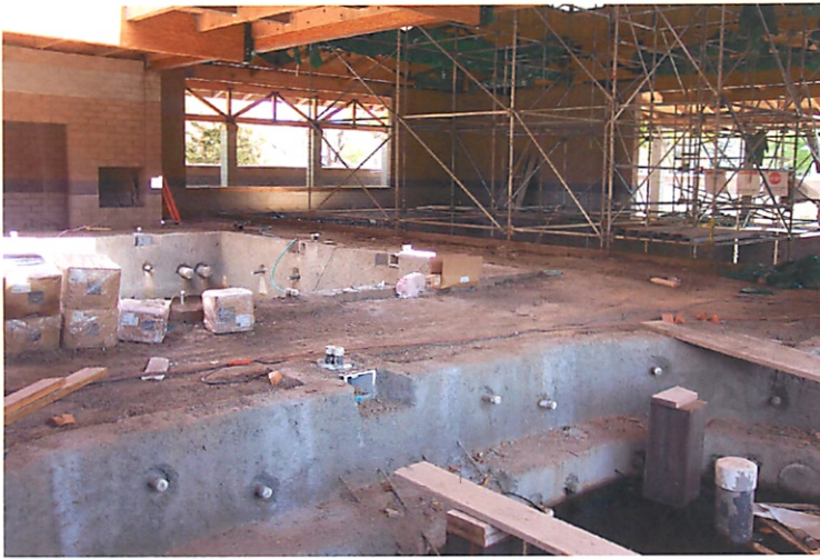
060511-037 New Senior Center swimming pool taken from west end looking toward giant hot tub.
