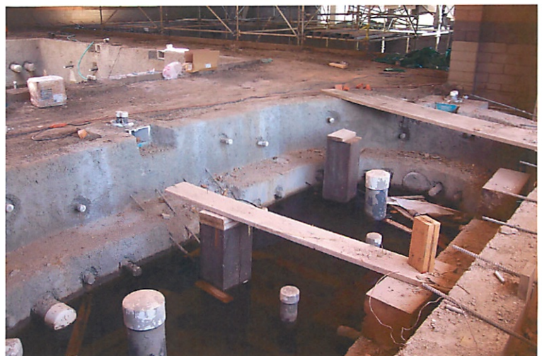
060511-039 New Senior Center swimming pool taken by Jacuzzi looking toward giant hot tub.
