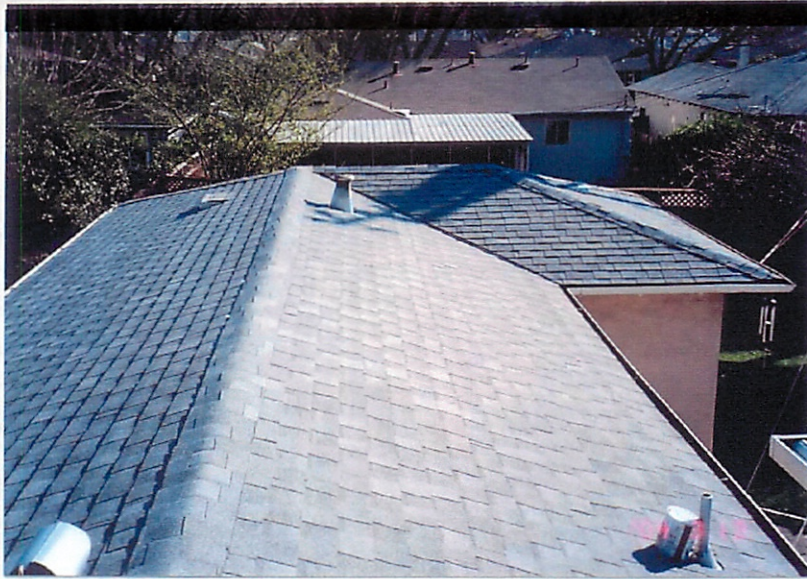
04-01-12 Looking over East Wing Annex at new roof on our house at 631 Kiely. 13 March 2004
