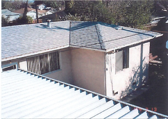
04-01-02 Looking at new roof on East Wing Annex of our house at 631 Kiely. 13 March 2004
