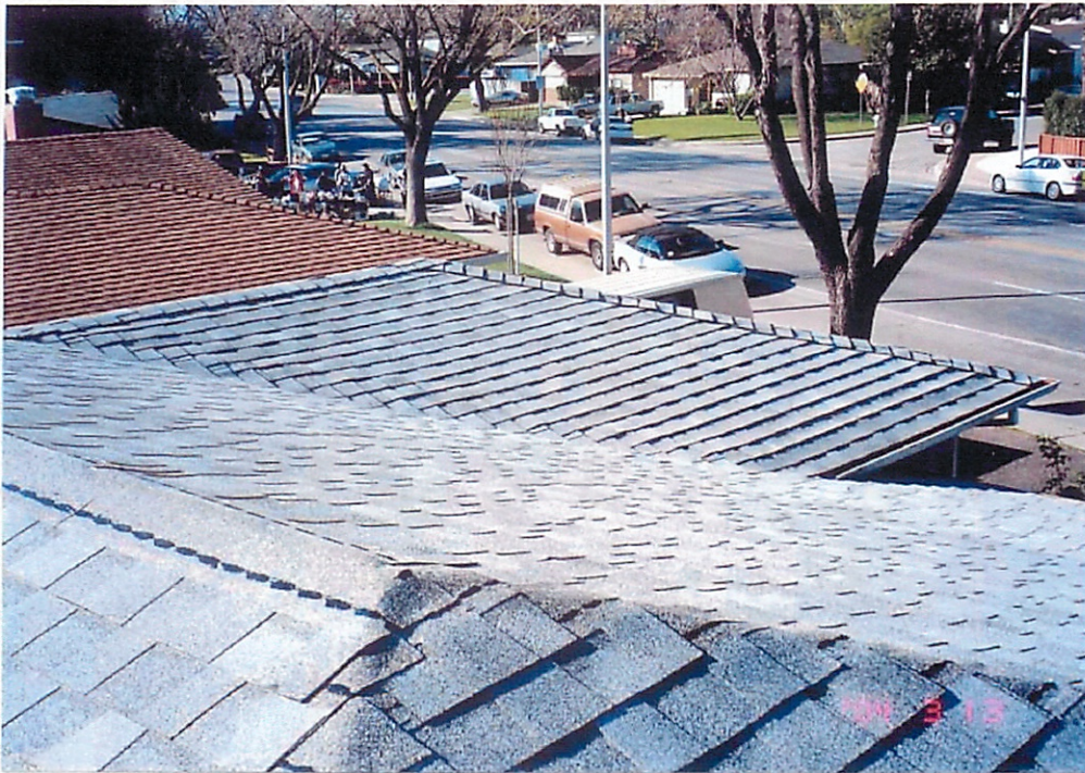
04-01-13 Looking over garage at new roof on our house at 631 Kiely. 13 March 2004
