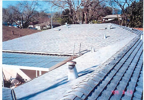
04-01-09 Looking from far end of East Wing Annex at the new roof on our house at 631 Kiely. 13 March 2004
