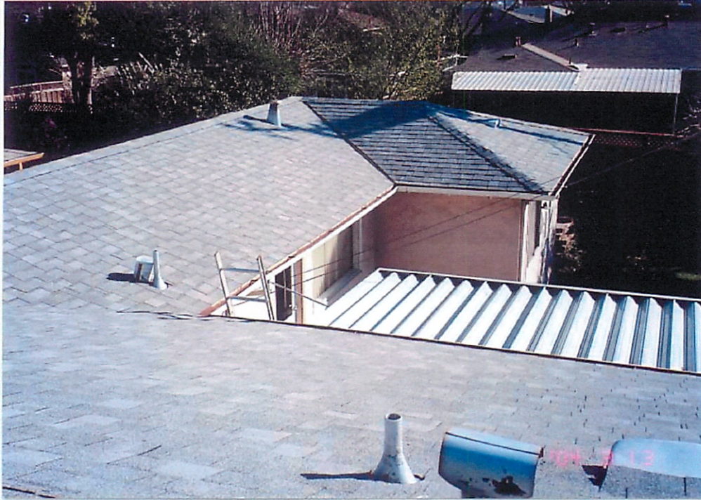
04-01-14 Looking over East Wing Annex at new roof on our house at 631 Kiely. 13 March 2004
