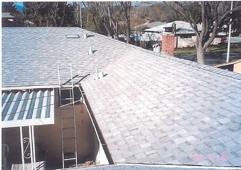
04-01-07 Looking from far end of East Wing Annex at the new roof on our house at 631 Kiely. 13 March 2004
